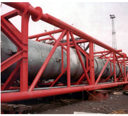
Suspension of gas turbine pipe 悬架的燃气透平机管道
